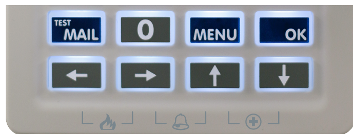
Figure 9: Keypad Emergency Alarm Trigger's
